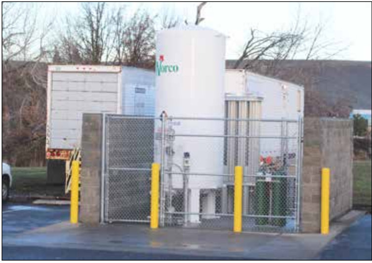
Photo by Michele Smith The oxygen plant supplies liquid oxygen for the Hyperbaric Oxygen Therapy chambers.
