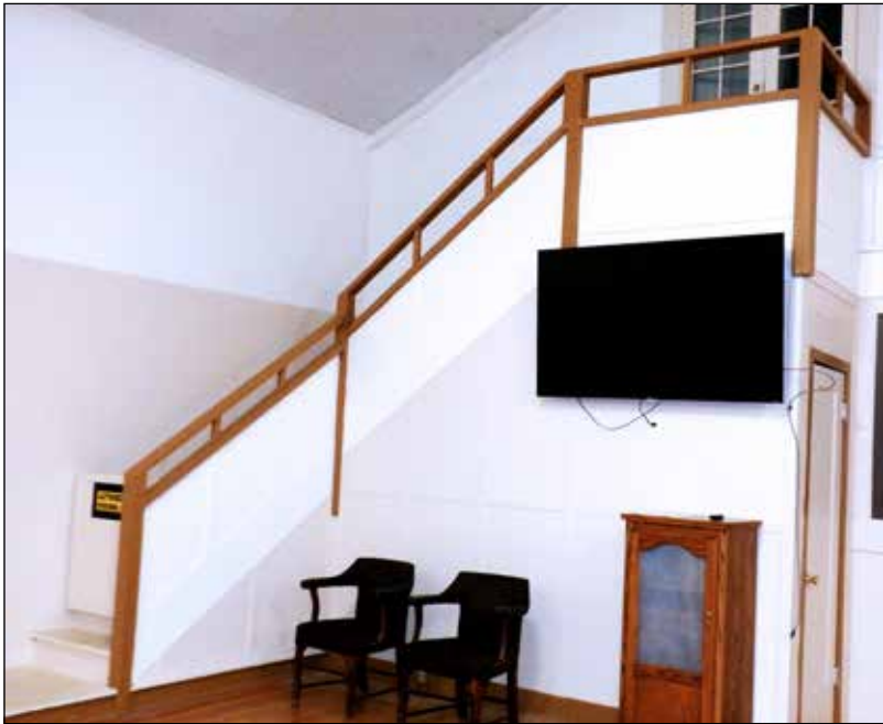
Town Hall board members Louie Gagnon and Allen Huwe built a higher and safer handrail going up the steps at Town Hall.
