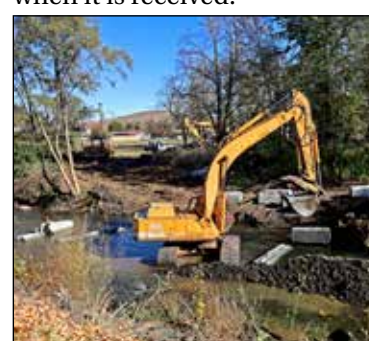
Photo by Beka Compton Crews from Harry Johnson Plumbing and Excavation used concrete barriers to divert water flow while repairing a damaged sewer siphon earlier this month. The siphon was damaged by heavy flood debris this February.
