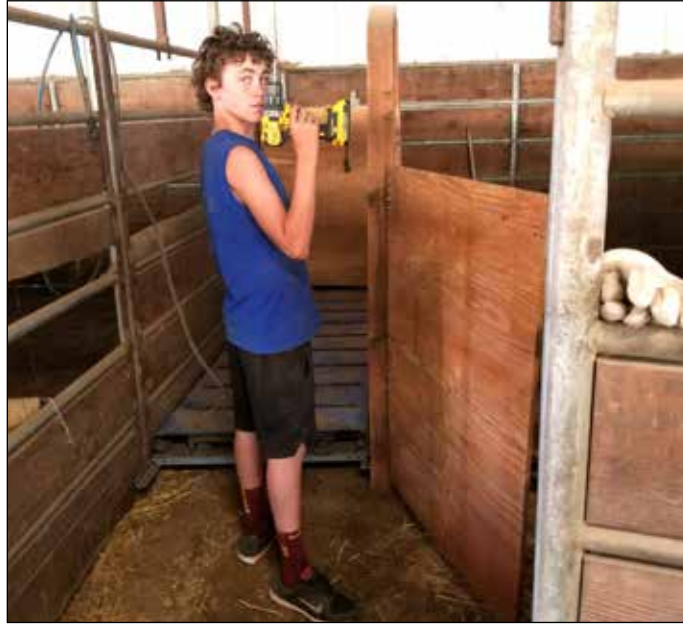
Photos Courtesy of Lisa Morrow Renovations continue on the newly improved livestock barn at the Waitsburg Fairgrounds. The latest addition includes a scale, donated by Guy McCaw. Duke Morrow framed and installed the scale with the help of Brayden Mohney (pictured) and Jay Dimak. "We owe all our supporters a big Thank you!" said Pen Pals 4-H leader Lisa Morrow.
