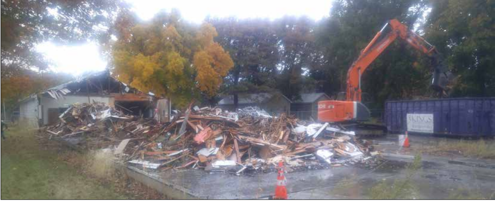
Photo by Ken Graham Demolition was well underway Monday at the former Seneca Activity Center, next to the county shop on the east end of Dayton. Columbia County took over ownership of the property earlier this year and will demolish most of the aging buildings there.
