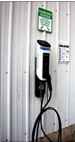
Waitsburg's new electric car charging station is situated across the street from Preston Park.
