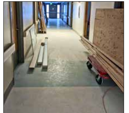
CCHS is remodeling the Booker Rest Home facility in preparation of the YWCA getting the keys in December.
