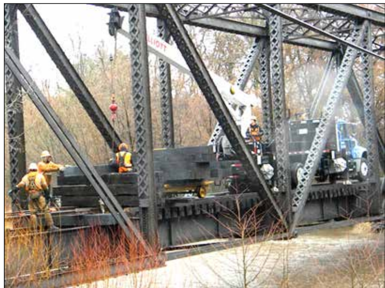
Crews repaired a railroad bridge between Waitsburg and Dayton earlier this year.
