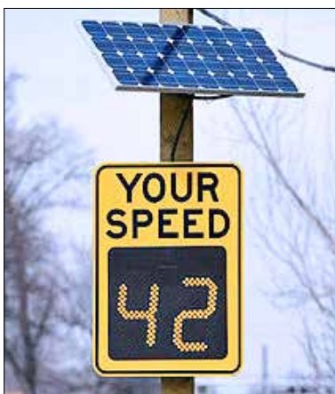
Solar-powered "slow down" signs will soon be posted at the three highway entrances to Waitsburg, courtesy of DOT funding.
